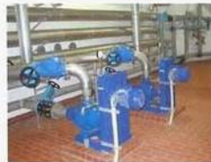
Heating Sludge Circulation Pump
