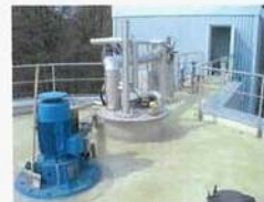
Head of the Digester
